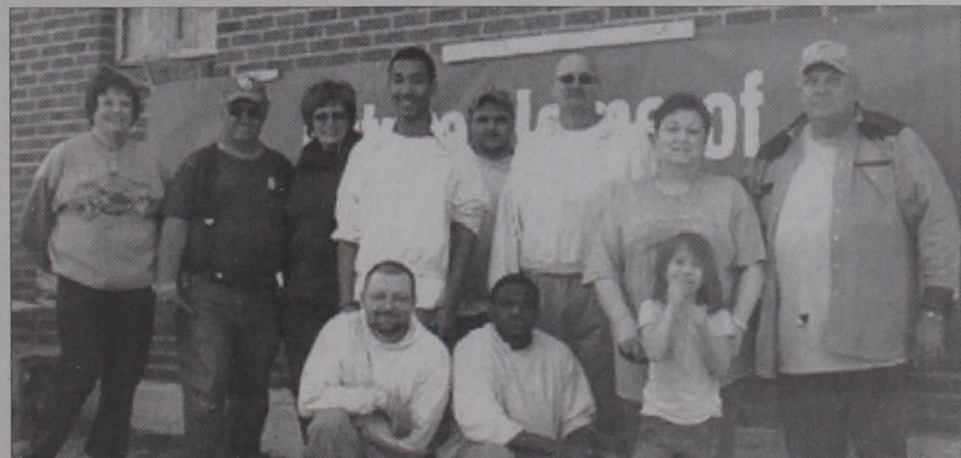
WORKERS: Volunteers began working on the Wheeler Historical Museum on Saturday, February 13, 2010. The group removed ceiling tiles and debris; plywood was put in place to protect workers from falling through the holes in the floor of the old Legion Hall. Pictured here are (back row, l. to r.) Bobby Hill, Leroy and Rhonda Meriwether, Mason Morales, Mauricio Lomas, John R. Nixon, Frankie Jackson, Jimmy Adams, (front) Shane V. Montgomery, James Morgan and Stormie Meriwether.
