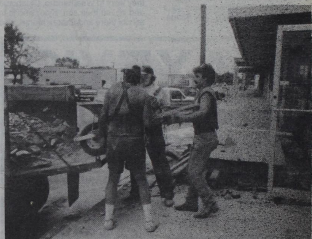
PROGRESS: The Rogue Theatre is being gutted to make room for the Oneighty Youth Center. The workmen here are shown loading one of several dump trucks loads of debris which was removed from the building. Opening of the center is scheduled for October 19, 1996.
