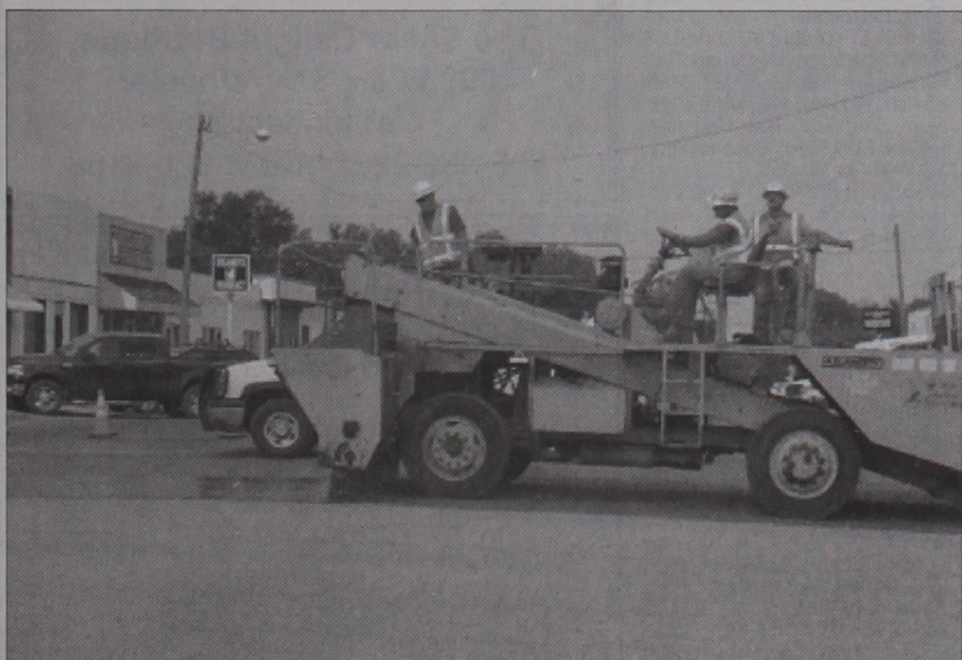
SEAL COATING: Wheeler's Main Street and 16 of the residential streets got a new layer of asphalt and gravel this past week. TxDOT workmen are shown here adding gravel at the corner of Main & Texas.
