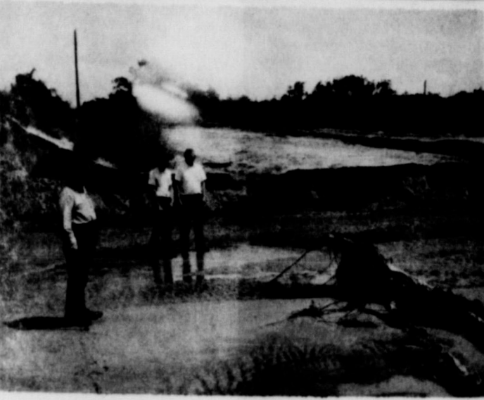
BAD, ALONG WITH THE GOOD: The rains Sunday night did a lot of good, but they were costly in the amount of damage to the county roads. Commissioner O. W. Pendleton (left) reported eight structures damaged in precinct 2. The wash pictured above is located three miles east, two miles north and one mile back east of Wheeler. The wash is 30 feet wide with cost of a temporary structure between $500 and $2,000. Two men with General Telephone Co. are shown uncovering the underground cable which was washed down stream. The men are Gale Gilbreath (left) and Bob Douthit of Memphis. — Wheeler Soil Conservation Photo
