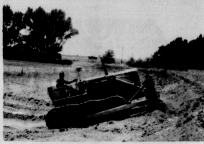
CONSERVATION CONTRACTOR AT WORK: Shown is a conservation contractor at work on a Diversion Terrace on the F. H. Davidson farm east of Wheeler. The Diversion will intercept runoff water from another farm and release it on rangeland where it will do no damage. The excess water was doing damage to a field of alfalfa. Technical assistance was provided by Soil Conservation Service personnel.
