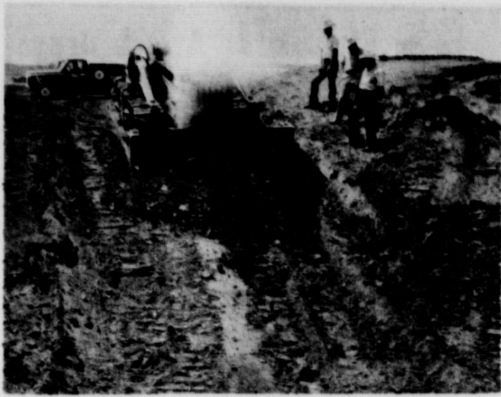
This picture shows some Soil Conservation Service personnel (L. to R.) Jerry Hefley, work unit aid; John Jackson, area engineer; and James Phillips, Conservation technician staking a concrete chute for a contractor to build on a grade stabilization structure for Mr. Jack Wardlow. This structure will prevent this gully from eating up across his field. If you have any erosion problem of any kind, contact your Soil Conservation Service Office in Wheeler.
