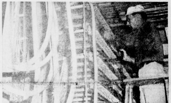
LABYRINTH OF WIRES - General Telephone Co. is completely revamping its telephone service here and between now and sometime this summer, all these myriad of wires, which go nowhere, will be connected before the service can be converted into seven-digit system. This is George Chapman, one of many who are working in the General building here, reworking the equipment.
