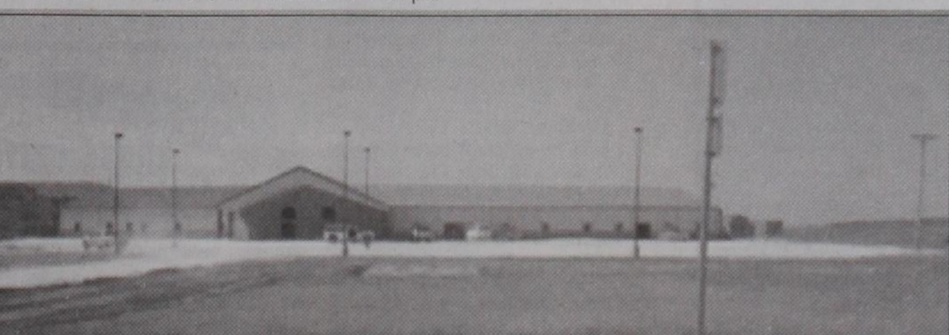
NEARING COMPLETION: The First Baptist Church on FM 2473 at the end of Main Street is set to be completed in August. The moving process is underway.
