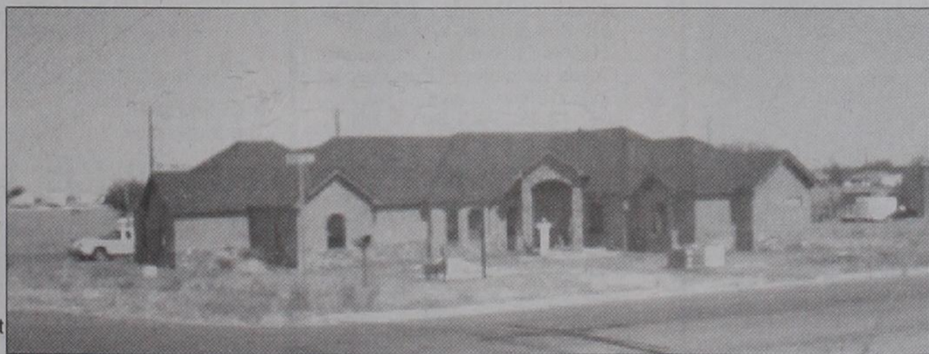
NEARING COMPLETION: This home at the corner of Mobeetie Street and FM 2473 is near completion. The builder is Ammons Construction of Pampa.
