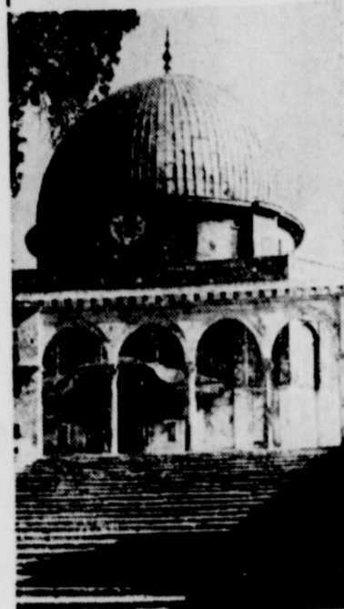
The famous Dome of the Rock in Jerusalem is undergoing repairs. The structure, pictured here, is being strengthened and the crust is being removed from the dome itself in preparation for a new coat of paint.
