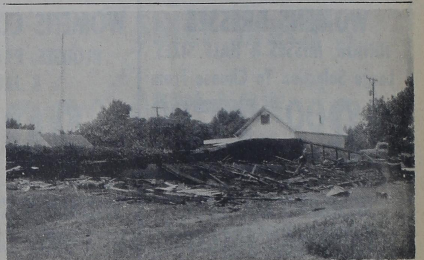
CLEARED AWAY: Work began last week to clear away the burned-out hull of a building in the 100 block of South Alan L. Bean Boulevard. It certainly helps the looks of the town when structures such as this are removed. Dan Luttrell owns this property.
