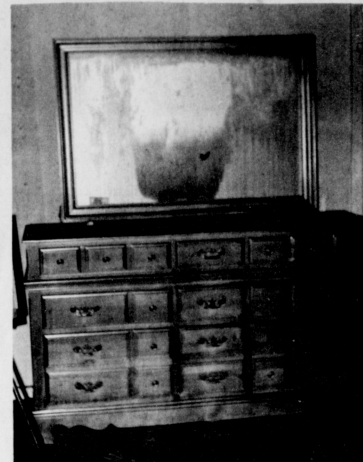
SMOKE-HEAT DAMAGE --Damage to rooms of the Gary Miller home by heat and smoke was severe during a Friday morning fire which started in the kitchen. This mirror is discolored and ruined by heat and a heavy film of black soot covers the entire house.
