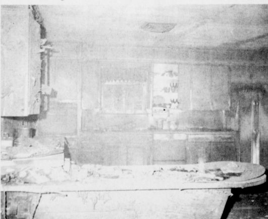
KITCHEN DESTROYED---Fire destroyed the kitchen furnishings and intense heat and smoke heavily damaged the home of Mr. and Mrs. Gary Miller Friday morning. This is what remains of the kitchen in the three bedroom brick home.
