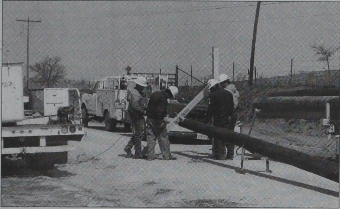
Greenbelt Electric workmen were out making repairs on Co. Road 3 Tuesday afternoon.
