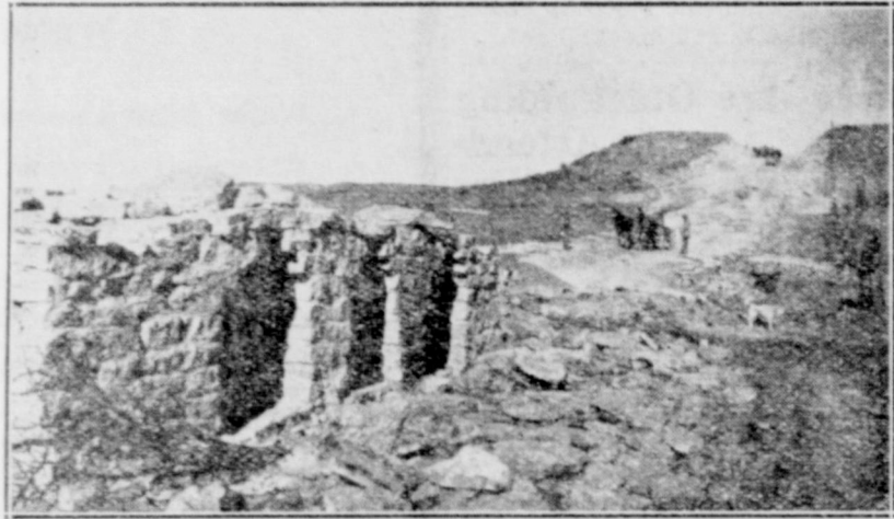
From this angle is seen the bridge and hill, with men and teams at work.
