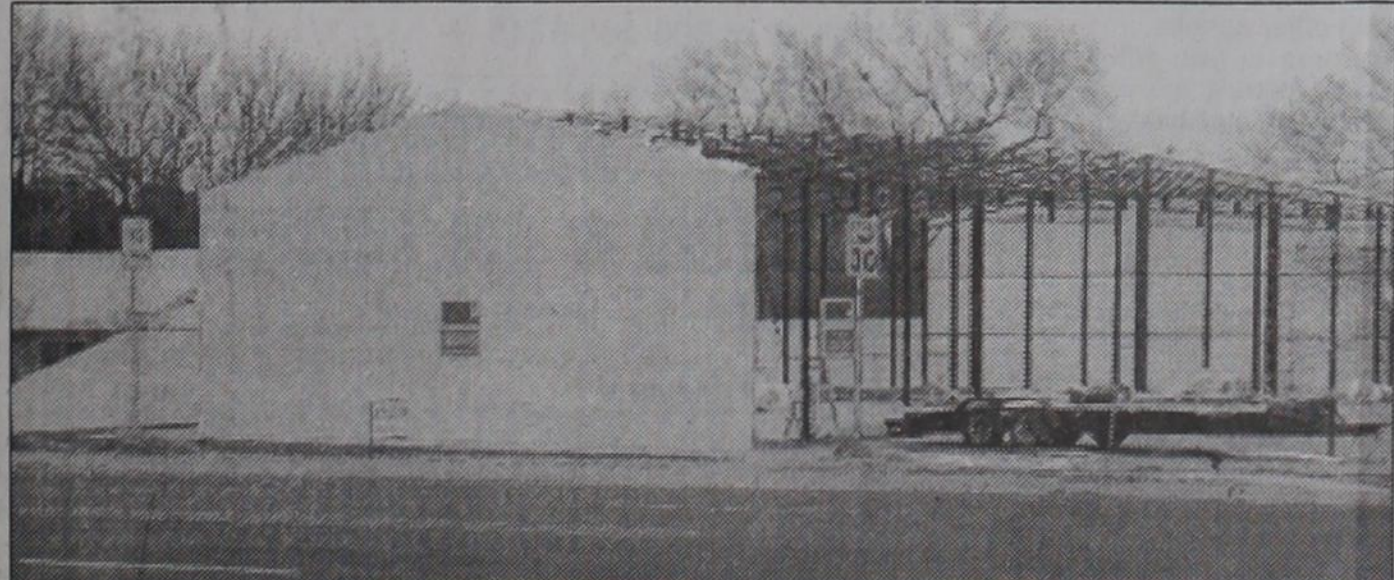
AMBULANCE BARN: Work is progressing once more on the new ambulance barn located at Seventh and Alan L. Bean Blvd. The building will have three ambulance bays. With opening in the south, the ambulances can pull onto either of the two streets.
