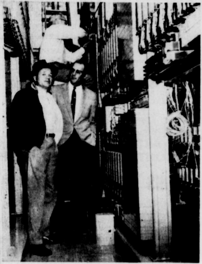
NEW TELEPHONE SYSTEM—Bill Walters, left, and A. D. Taylor, right, of Southwestern Bell Telephone Company, make a final check of Eastland's new dial switching equipment which will go into service at 1:01 a. m. Sunday.
