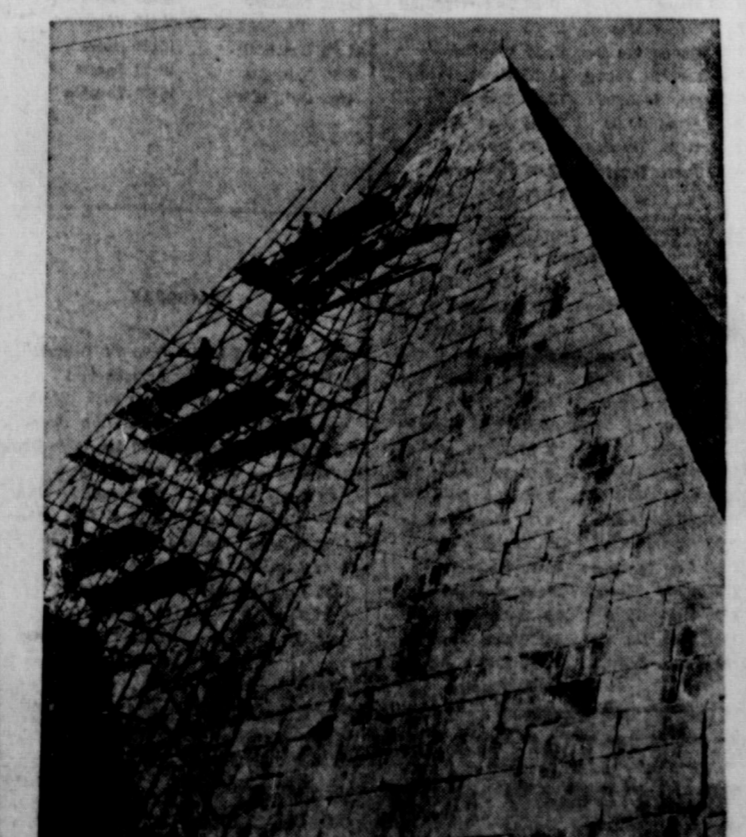
POINT OF VIEW—Workmen make repairs, not on the Egyptian pyramids, but on the tomb of Caius Epulo, in Rome.
