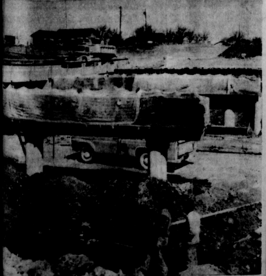
'WORK' — Construction of the bridge to span the Leon River where Highways 101 and 102 are crossing is moving fast. Pillows and most of the sub-surface cement work is completed. At left, top, a dump truck can be seen crossing the old bridge. Construction Co. of Plainview is subcontractor to Cooper and Woodruff Inc., contractors, for the bridge work. (A&C Photo)
