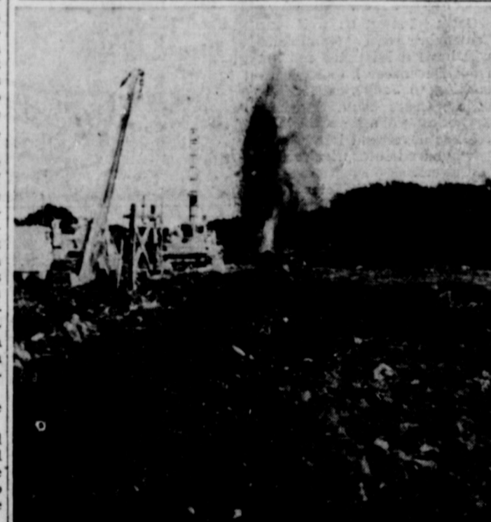
ROCK, DUST and dynamite powder go sky-high as Lone Star Gas Company pipeliners blast through solid rock to lay the 14-mile, 16-inch pipeline stretching from Gordon to Sweetwater. By mid-November, the line had reached a point north of Ranger. Approximately 1000 feet of pipeline right-of-way is "shot" at a time, with three sticks of dynamite being placed in holes 36-inches apart.
