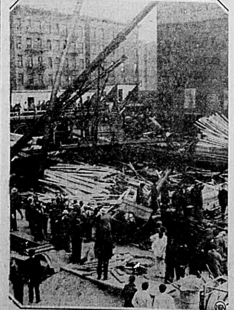
NEA New York Bureau Here is the jumble of wreckage in which two men died and a score were injured when a building under construction collapsed in New York. Tall girders are shown tilted in the air at crazy angles—one is slanted obliquely against the walls of an adjoining factory—after the steel framework of the four-story structure had crumbled and crashed, trapping some of the workmen underneath. An investigation of the accident was ordered.
