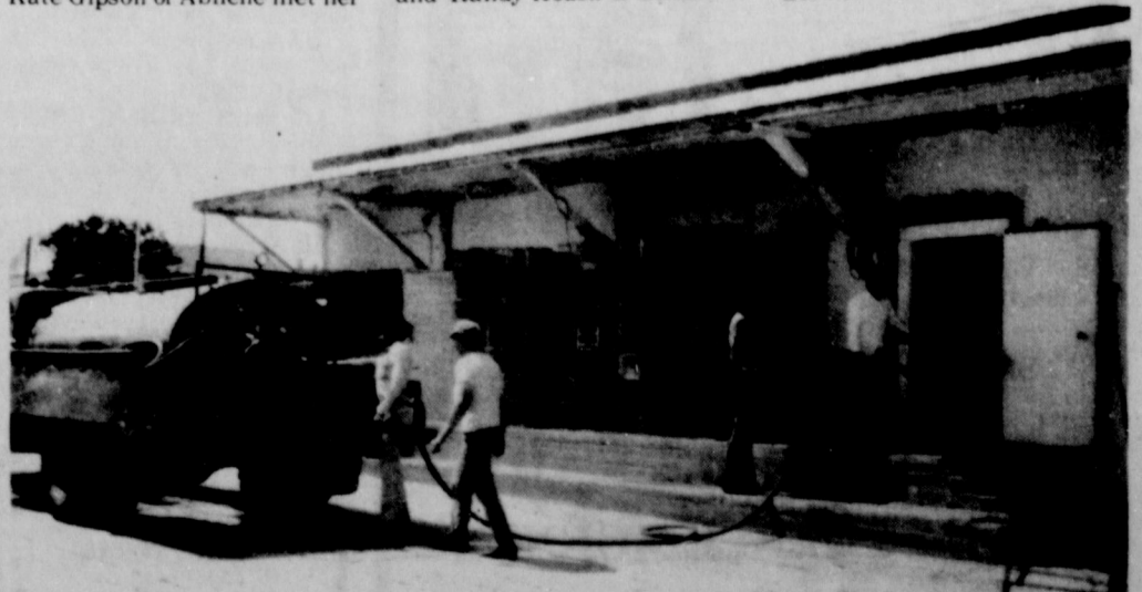
NOONTIME FIRE which erupted at the Foremost Dairies Storage House shortly after 12 Tuesday left the building damaged at 1:30 after Volunteer Firemen stamped it out. Estimates are that damage would exceed $500. There were no injuries.
