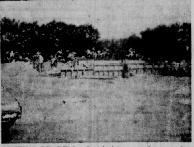
GETTING READY for foundation pouring are two house sites on just-opened S. Ammerman St. in the newly-developing Valley View Estates.
