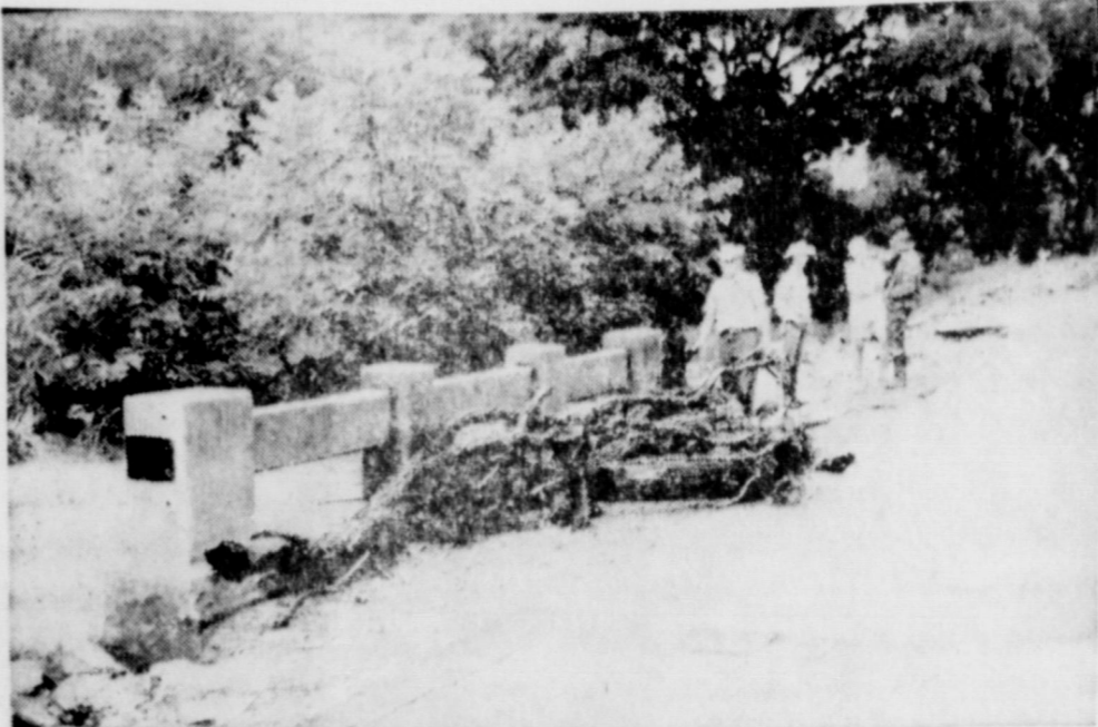
BRIDGE DAMAGE — Debris and damage abound at this North bridge on U.S. 183 south of Cisco. Kent Word of the area said, "This is the highest I've seen the water in 83 years." The east shoulder was washed off. Among those shown are Rayford Young of the Soil Conservation office. The Bill Wende property adjoins this area and was flooded. (All water pictures made by John Simpson of the Eastland SCS Office with Staff Processing by the Telegram)
