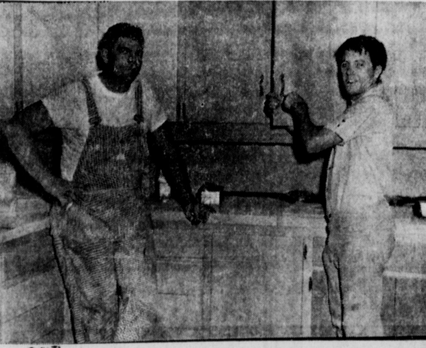
STALLING NEW KITCHENS — John Foster and Mike Siebert were busy installing four new kitchen units in the high school home economics department today, updating the facility which was originally installed in 1927. Other fix-up projects are underway in preparation for the Sept. 1 opening of schools here.
