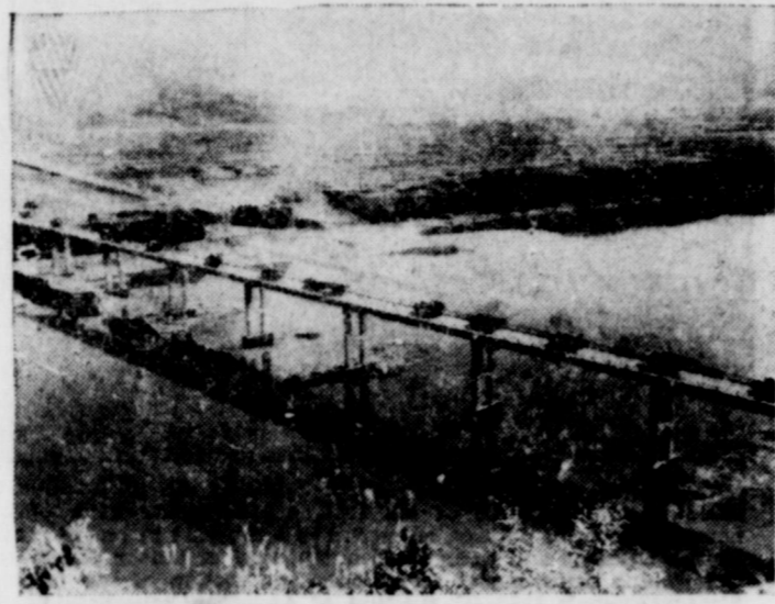
BUILT UNDER ENEMY FIRE, Libby Bridge spanning the Imjin River in Korea was completed by U.S. Army Engineers in five months, 21 days. The 1,074-foot span was named for the late Sergeant George D. Libby of Linden, N.J., winner of the Medal of Honor. The 8th Army Engineer Construction Battalion was awarded the Republic of Korea Presidential Unit Citation for building the bridge.
