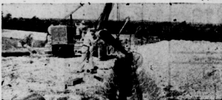
PIPELINES —a network of long distance pipelines is necessary to bring the natural gas from its origination point to the city where it will serve uninterrupted, day and night.
