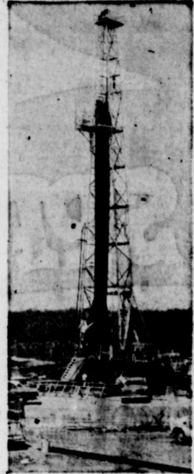
DRILLING —After geological explorations are made, leasing completed, the rig is positioned and drilling begins. Drill bits bore deep into the earth to possible natural gas strata.
