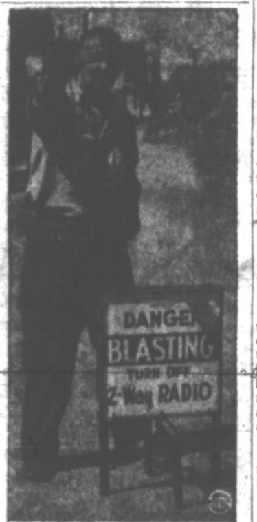
TURN IT OFF —Construction crews in York Beach, Me., don't mind radio programs or conversations on two-way radios. They put up this warning sign because dynamite can sometimes be set off by the radio signal of a passing car. Some frequencies have reportedly set off a charge prematurely as far away as 400 feet.
