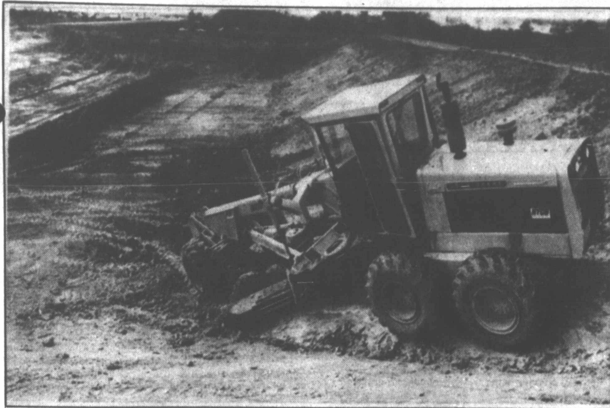
A grader scrapes dirt at the 294-acre site of the Big Hill Petroleum Reserve Project in Winnie. The site is one of six being built nationwide that will eventually provide storage for 140 million barrels of crude oil in 14 caverns hollowed out of underground salt domes. When complete the project will have a warehouse, a laboratory and fire station, a security building and an office building. All storage will be underground. (AP Laserphoto)
