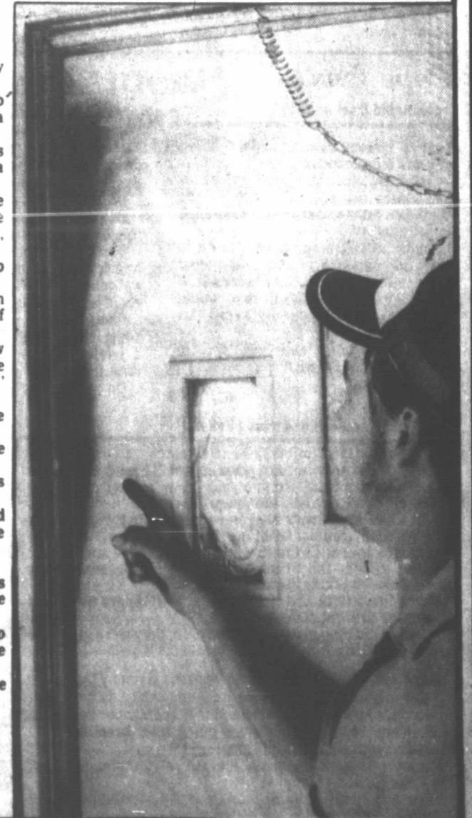
Jerry Finney points to scorch marks caused by a lightning-strike fire that damaged his rural home. (Staff photo by Bruce Lee Smith)
