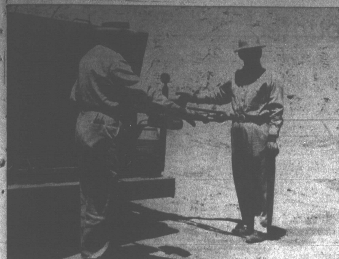
LOWERING A CHARGE — O. E. (Chennie) Chenoweth, left, carefully watches his line lowering a shell filled with solid nitroglycerine into a well on the Reynolds lease seven miles south of town.
