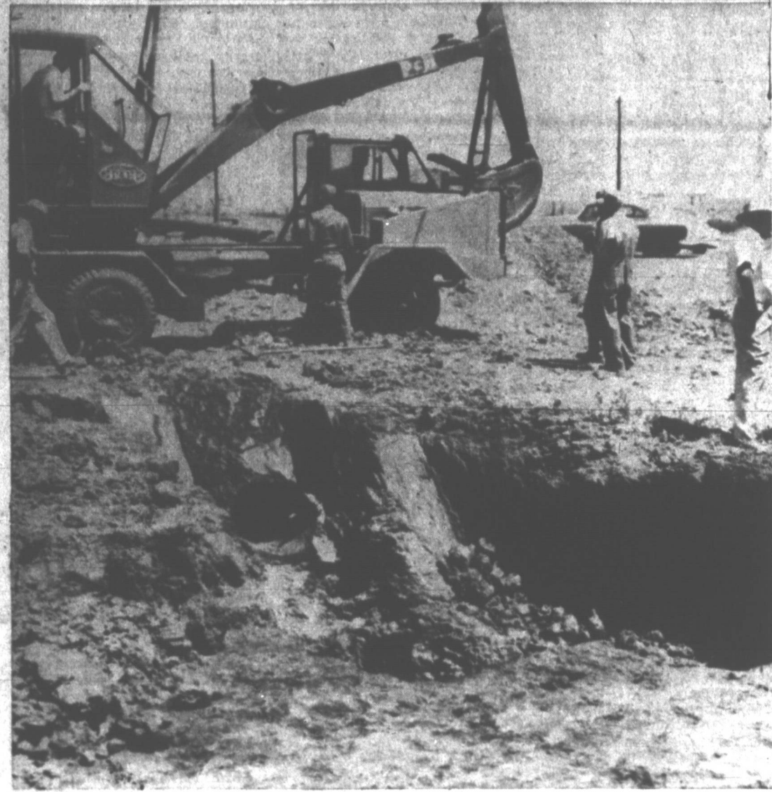
BLOWN OUT - In the center foreground is the 20-inch Cities Service gas pipeline which "blew" early Saturday afternoon. In front, and to the left of the line, is the portion of earth torn up by the blast. To the right of the pipeline is where the back-hoe (in background) had been working. (News Photo)
