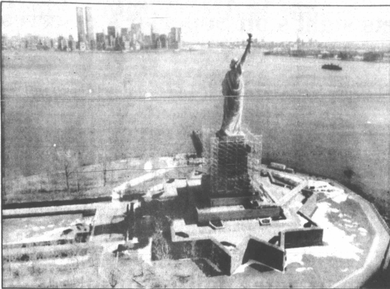
RESTORATION CONTINUES —The Statue of Liberty restoration continues Monday in New York in preparation for the monument's 100th anniversary in October 1986. The work is scheduled to take 30 months and cost about $39 million. (AP Laserphoto)
