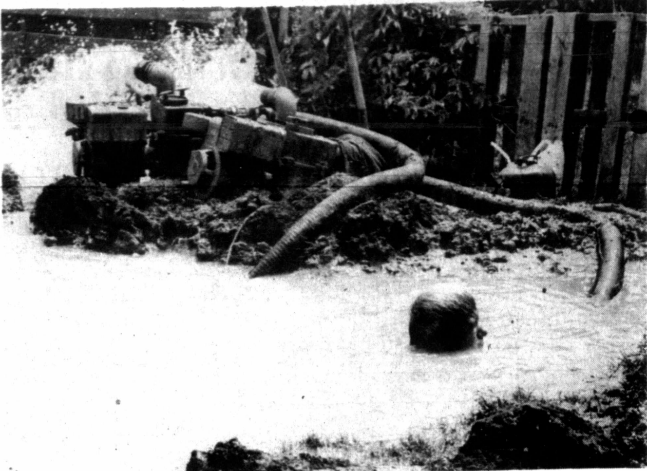
NECK DEEP-A city of Pampa employee looks like he's swimming for his life. But he's actually trying to get to a broken water pipe in the alley between Hamilton and Williston Thursday afternoon while a pump in the background flushes water out of the hole. The break in the four-inch line flooded the area. (Staff photo by Ed Copeland)
