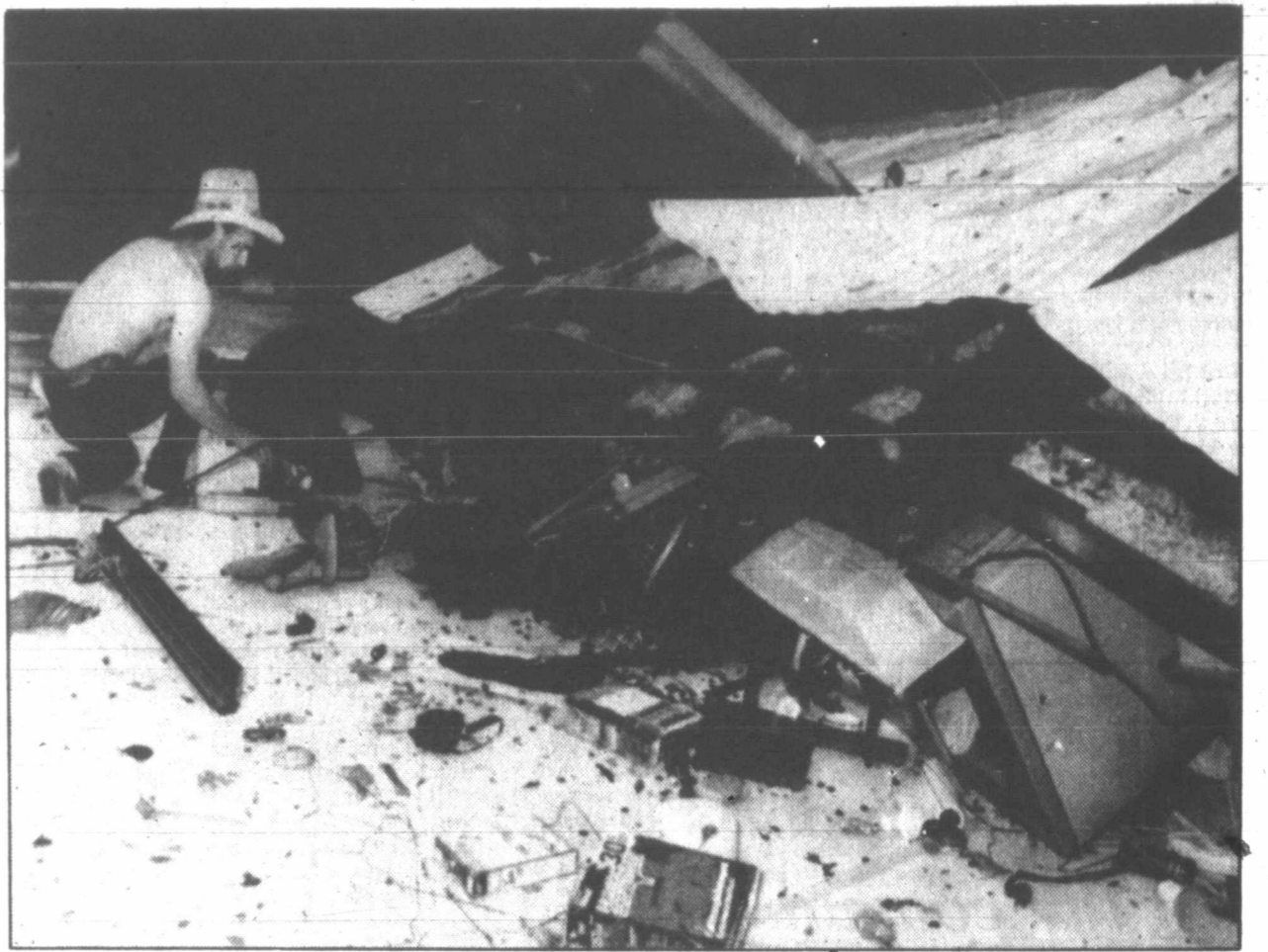
WIND DAMAGE—Bill Brasher and his brother Dan look over the damage to their mobile home in Garland, a northeast suburb of Dallas. Although no tornadoes were
