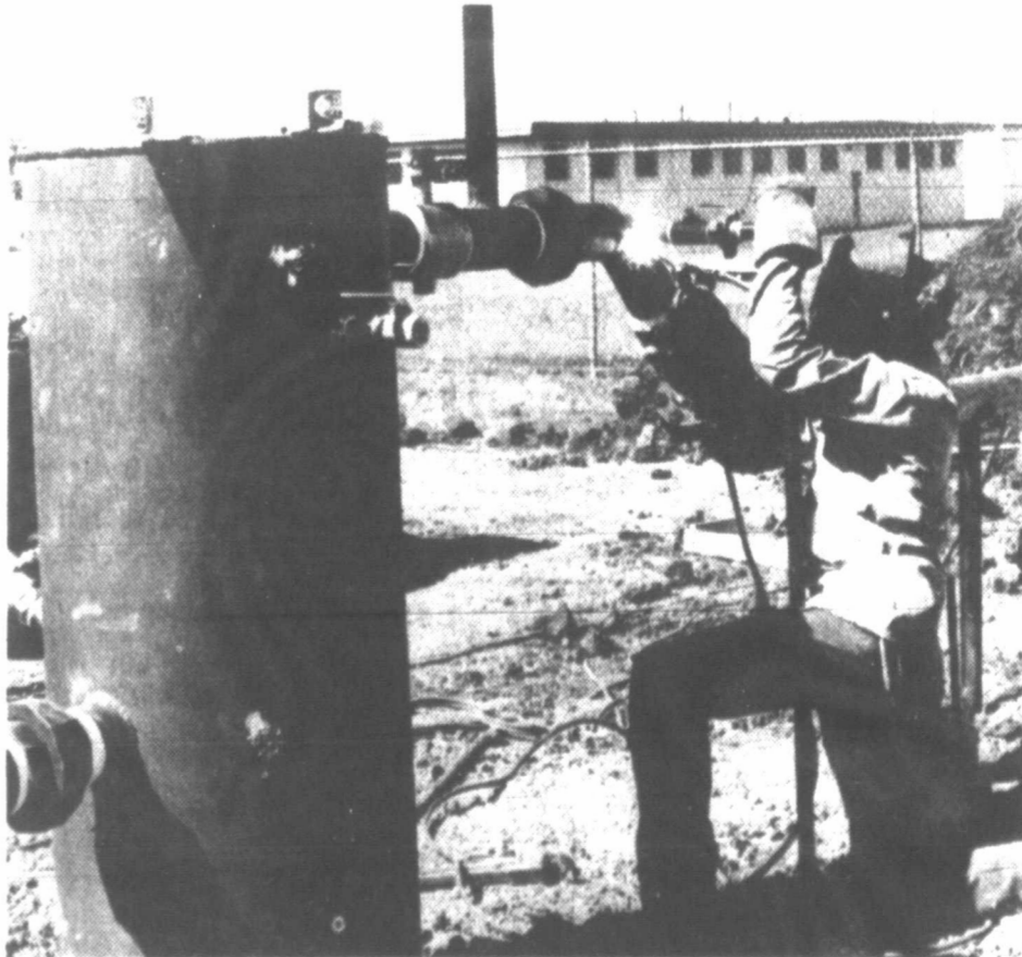
NEW GAS WELL — A White Deer city worker welds the piping of a new gas well near the White Deer High School stadium. The well is part of the city's municipal gas system. It is the second well to be connected to the system. (Staff photo by Cathy Spaulding)
