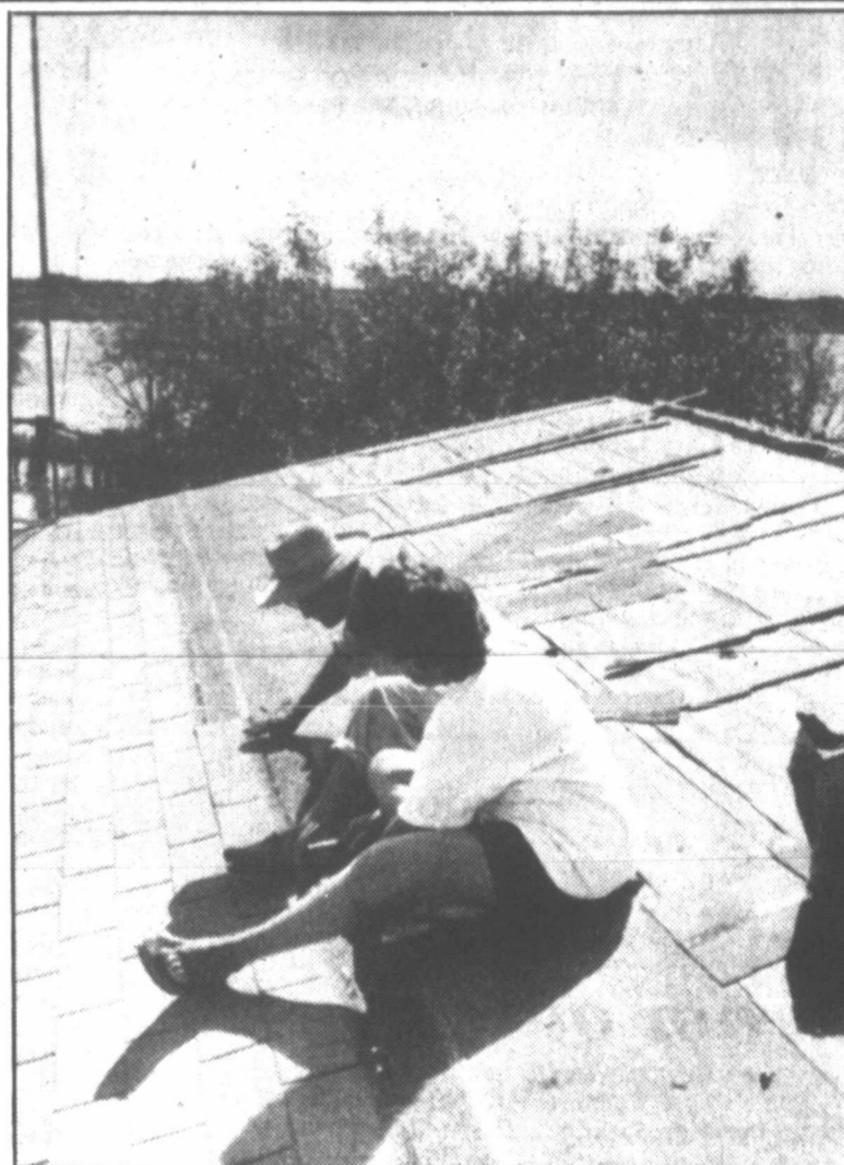
CLEAN-UP CREW—Tinoteo and Marie Davila work on the roof of their home north of Harlingen repairing a roof blown off by storms that flooded the eastern Rio Grande Valley last week. In the background new rain clouds form, but forecasters said the torrential downpours are over.
