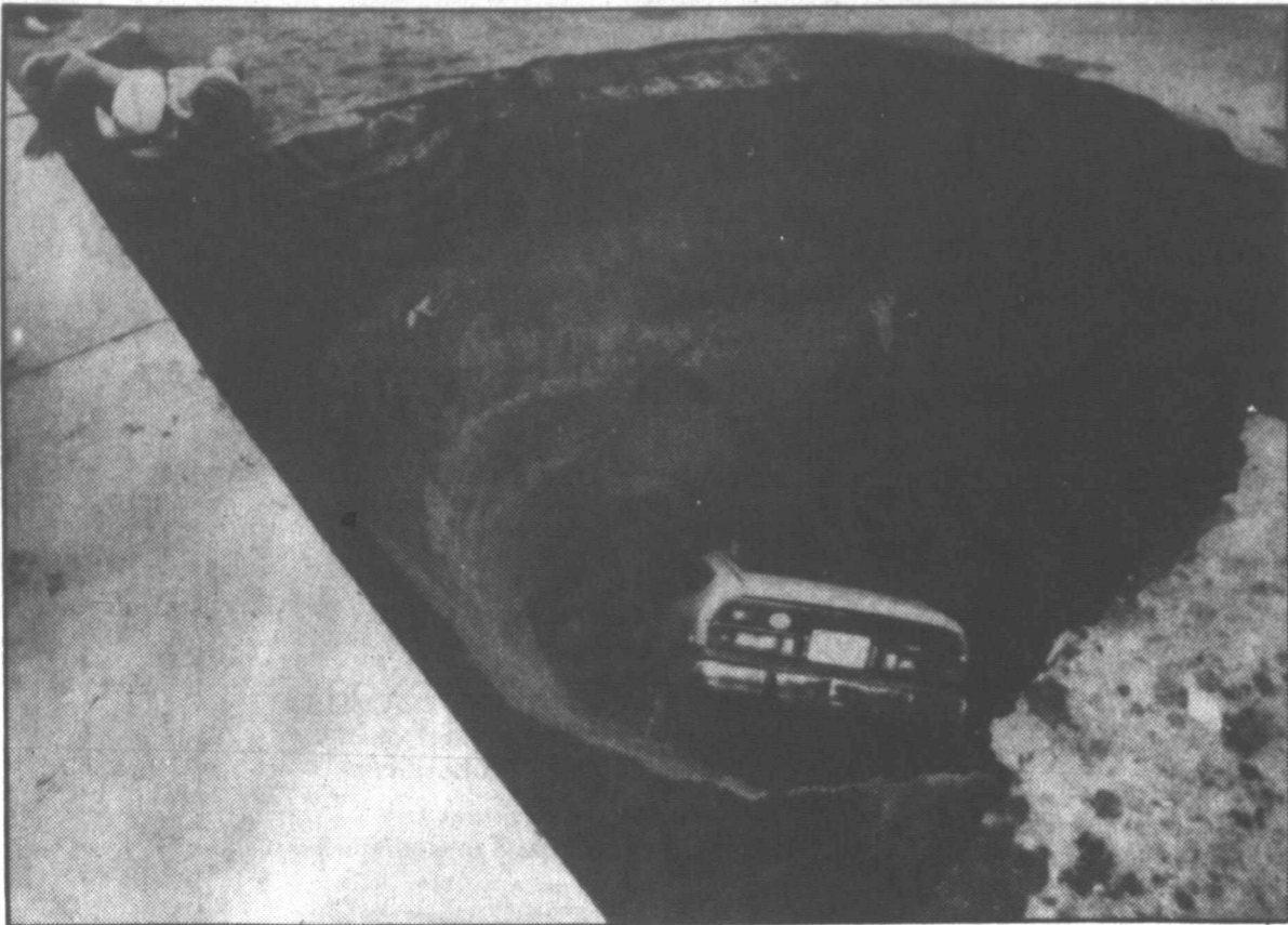
HUNGRY HOLE —Augusta, Ga. fireman Melvin Harris peers into a 30-foot hole which swallowed the car of Augusta Chronical newspaper carrier John Sammons while Sammons was on his route Tuesday. City officials said the collapse was apparently caused by a leaking storm sewer which had slowly washed away the soil beneath the parking lot where the cave in occurred. (AP Laserphoto)
