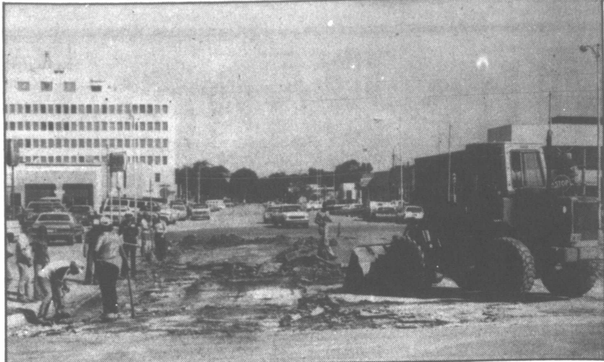
TAKING TO THE STREETS —Crew members for Lewis Construction Co. work on the summer street repair project Wednesday at South Somerville and Atchison streets in front of The Pampa News office. The crews have moved into the south sections of the city to repair potholes
