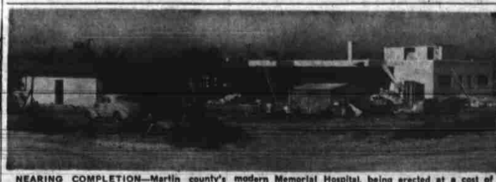
NEARING COMPLETION—Martin county's modern Memorial Hospital, being erected at a cost of $210,000, is entering the finish stage of construction. Now 75 per cent toward completion, partitions are being installed, wiring completed, and the finishing work launched.
