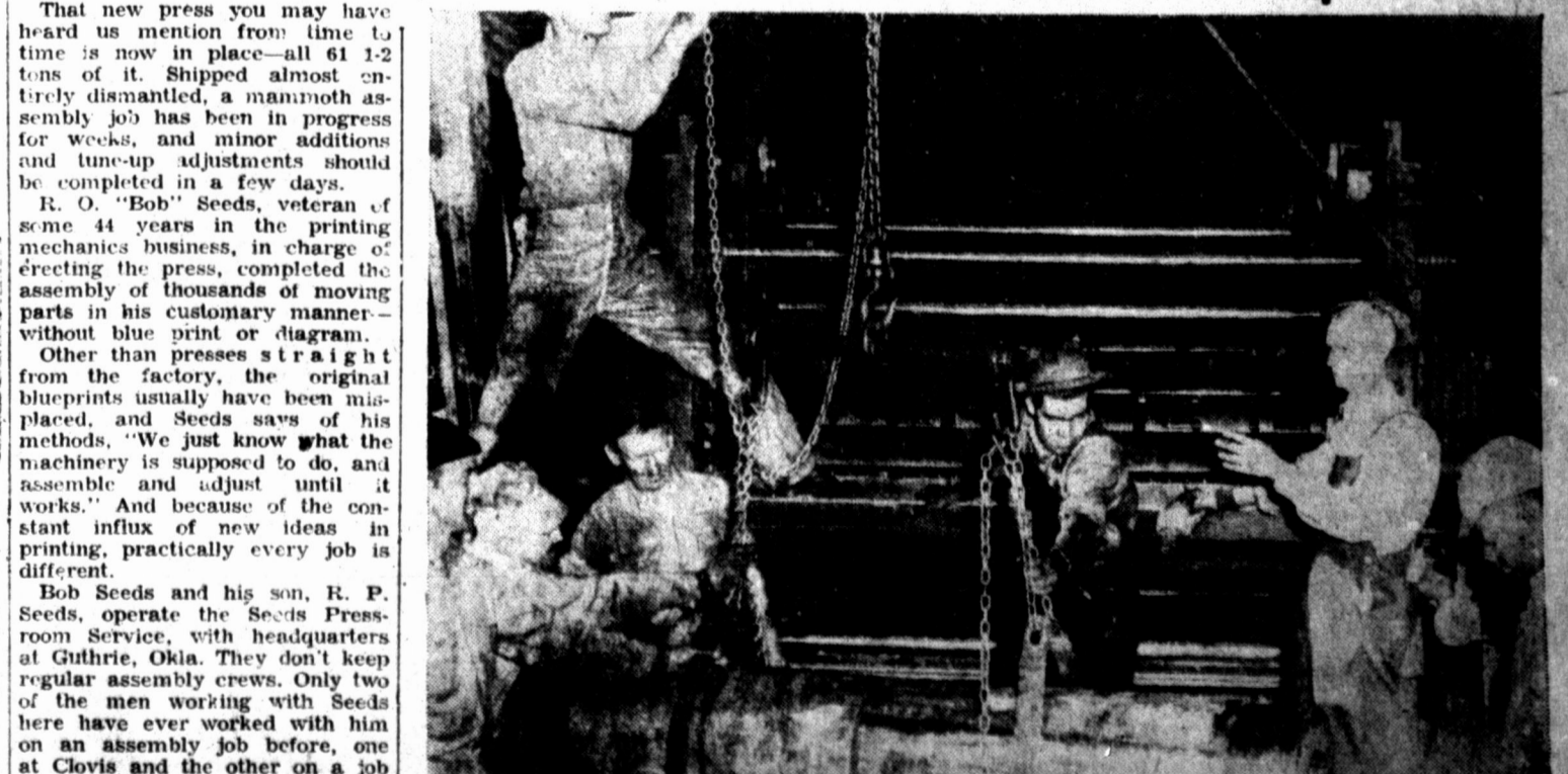
PRESS INSTALLATION—R. O. "Bob" Seeds, second from right, directs assembly of the new press being installed at The News. Above: Ralph Walker of Pampa. Left to right: Ray Parks of Pampa, G. L. Martin of Kansas City, Elmo Heibert of Pampa, Paul Porter of Pampa, Bob Seeds of Guthrie, Okla., and John Ransom of Clovis.
