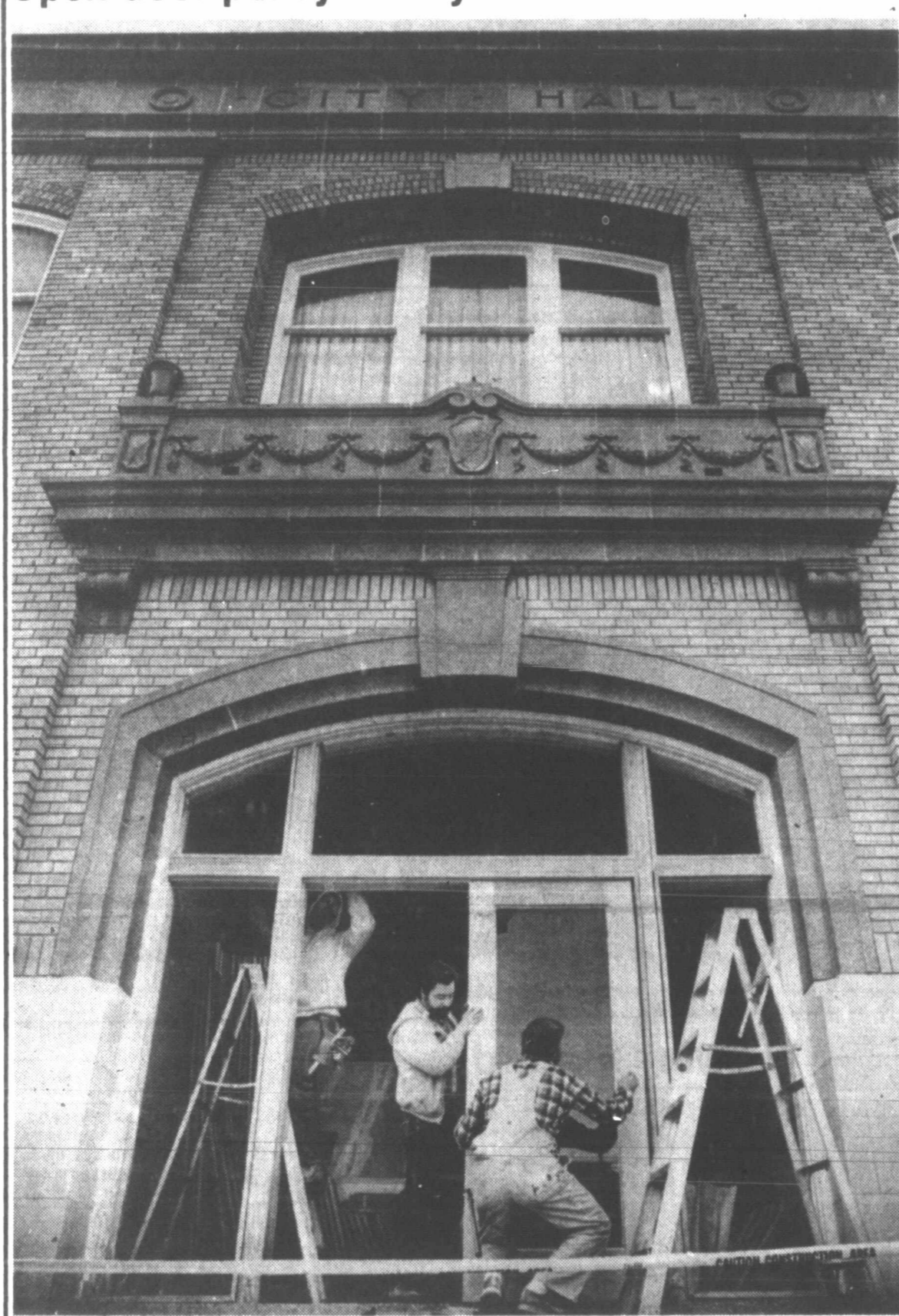
City crews fit a new door for the north exit of City Hall Friday, part of the continuing renovation of the building housing Pampa city government.
