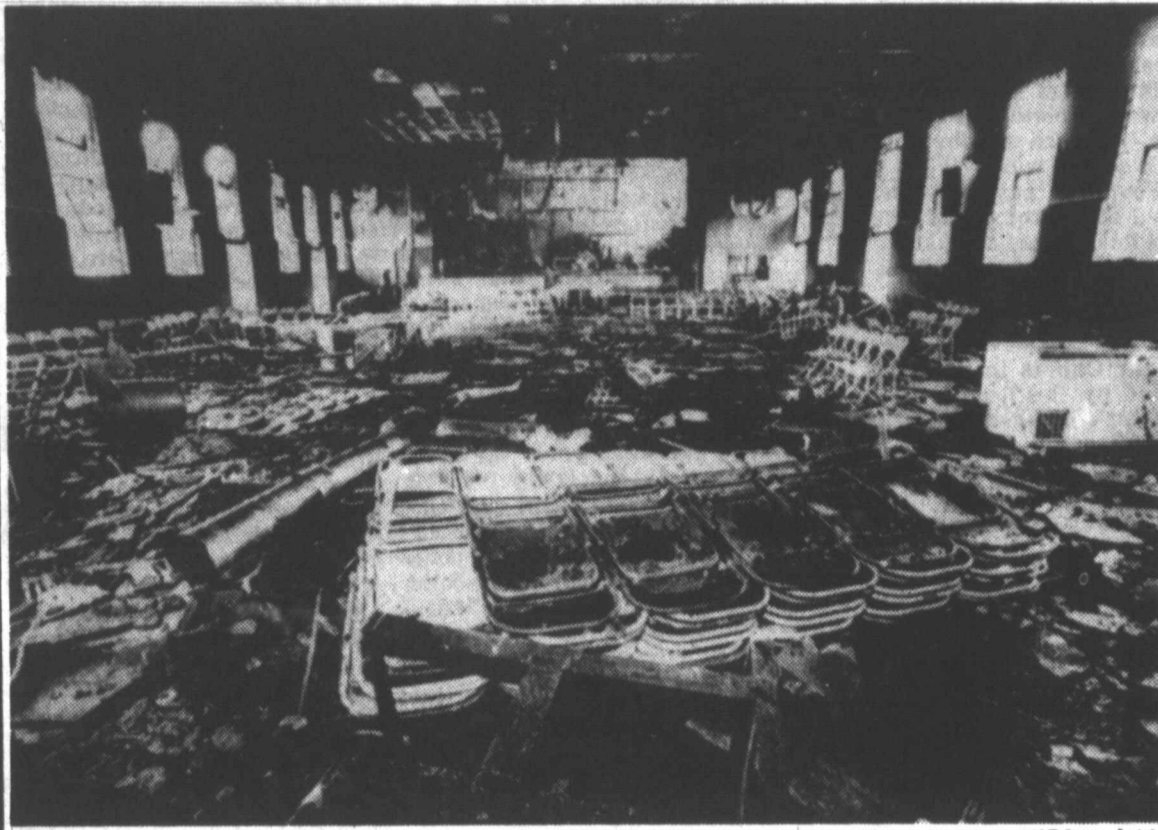
This is the inside of the auditorium at the State Correctional Institution of Pittsburgh after a four-alarm fire destroyed it Tuesday.
