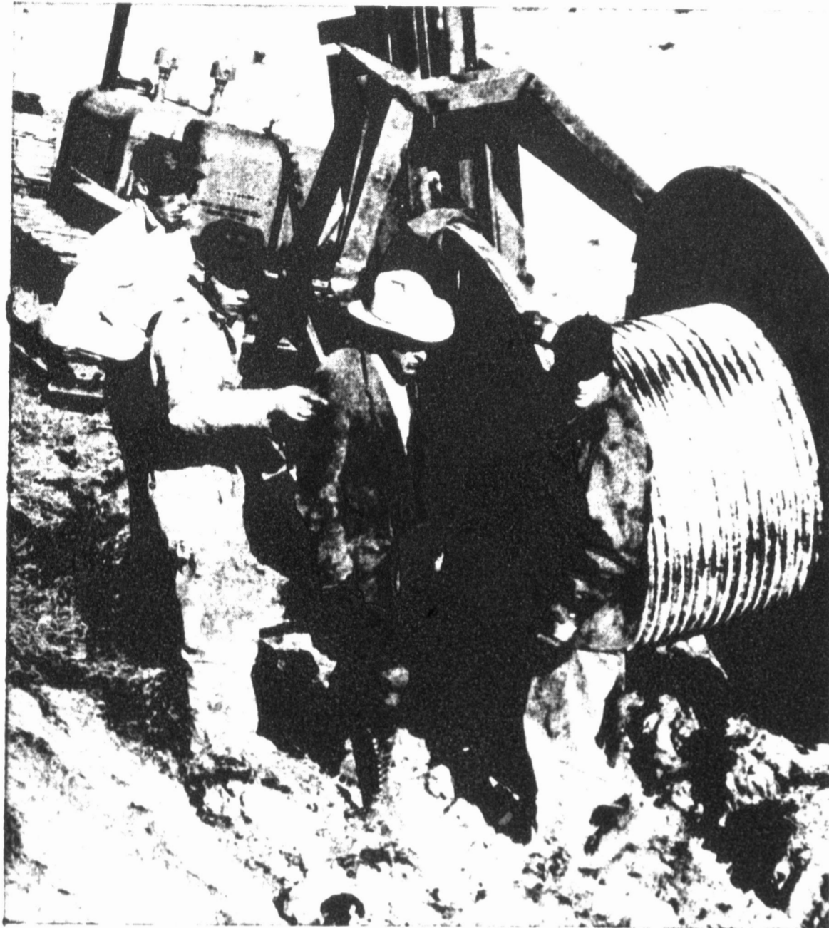
BURYING THE CABLE - Workmen for the Lewis Excavating Co. of Dumas shown here burying the cable which will help bring the dial telephone service on an inter-city basis to Pampa, Borger and Skellytown. So far, seven miles of cable have been buried 40 inches deep. (News Photo)
