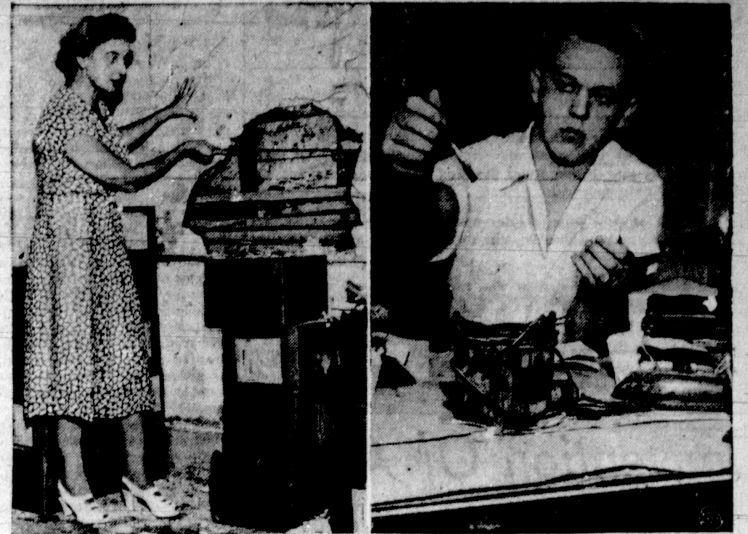
REASON FOR A CHANGE —Here's why the U.S. Passport Office is moving into new quarters in Washington, D.C. In photo at left, Director Frances Knight knocks a piece of plaster off the almost crumbling walls of the Civil War-era building now housing the Passport Office. Boxes on floor contain dead files which have to be stored in the basement because there is no room for them in the office. At right is a staff member pasting photos onto passports, using an archaic glue pot and hot irons which press the picture onto the passport. This old, time-consuming method will be streamlined in the new building.
