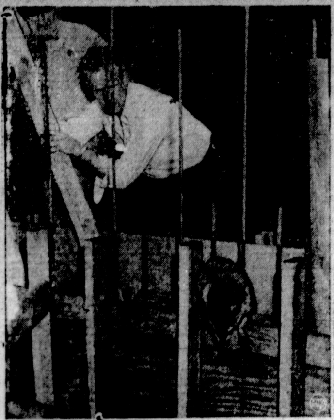
OBSTINATE RACCOON —This stray raccoon stood up for its rights in Washington, D.C., despite the day-long proddings of workmen, police and passersby. The 'coon was found holed up in the narrow 15-foot-deep forms that were ready for concrete pour- ing for a transformer vault at the rear of the Capitol. It refused to be dislodged and stayed until night and departed under cover of darkness—as it had come.
