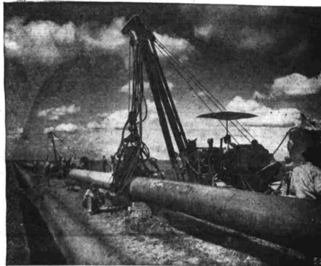
WELDING BIG PIPELINE —A crew with a pressure welding machine hooks up some of the Texas sections of the 1,265-mile pipeline of the Tennessee Gas & Transmission Co., to bring natural gas from Corpus Christi, Tex., to Charleston, W. Va.
