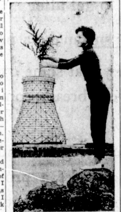
CAMERA MAGIC —Mrs. Jack Hess of Hamburg, Germany, demonstrates how to tell a "tall story" as she reaches over to place a bouquet in a modernistic "flower vase." The "vase" is actually a 150-foot water tower under construction in the distance.
