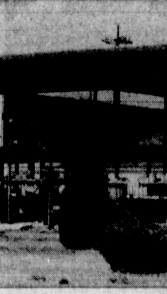
MAKING PROGRESS—Construction work on the new office building at the Cabot Shops, west of Pampa, is well underway with the steel work completed and the brick walls about one-third completed. The building should be completed by September 10 and some of the offices will probably be in use by September 1. Cabot officials report. The new office is being constructed, along with a new shop building, to allow room for personnel from Franks Manufacturing Company, a Cabot subsidiary, to move here about September 1. (News Photo)
