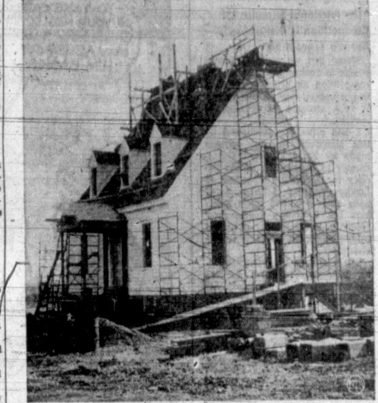
THIS OLD HOUSE IS NEW—Under construction in Charlottesville, Pa., is a replica of the house called Shadwell where Thomas Jefferson was born. The site is not far from Monticello, Jefferson's famous home. Built in the 1730s, the original Shadwell burned down in 1766.
