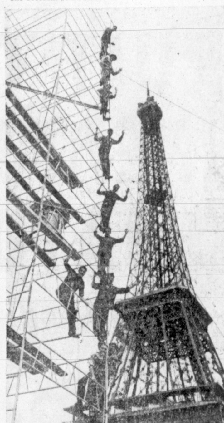
GOING SOME —Getting up in the world, workmen pose acrobatically atop a tall scaffolding on the left bank of the Seine River near the Eiffel Tower in Paris. They were erecting a powerful beacon light for a Nautical Show, which was officially opened by President Coty.
