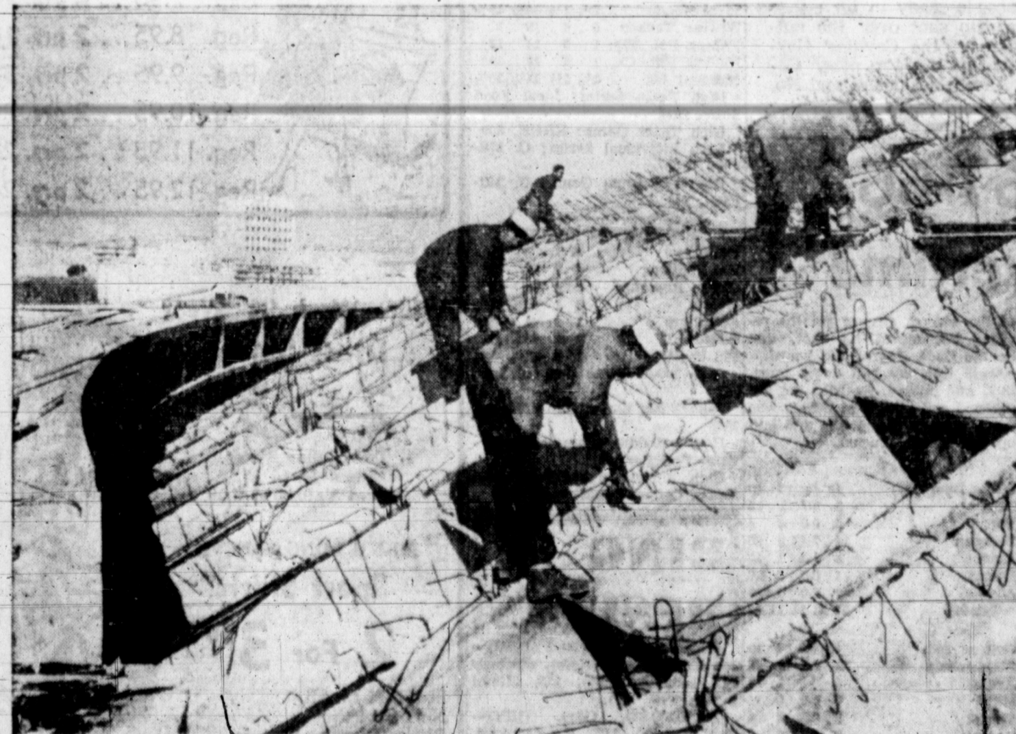
EVER UPWARD —As workmen in Rome tighten the supports atop the upper section of the sports palace being constructed for the 1960 Olympic Games there, they somewhat resemble mountain climbers. A mammoth dome more than 300 feet in diameter will top the structure which is expected to cost more than three million dollars when it's completed.
