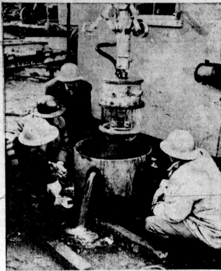
LOOKOUT, BELOW—Engineers study a special underwater television camera at a construction site in Boston. The camera was designed to be lowered to the bottom of a 30-inch, pipeline steel caisson, some 140 feet below surface level. Caissons, 144 of them, will support a new 52-story office building. The picture relayed by the camera shows the rock formations at the bottom of the caissons.
